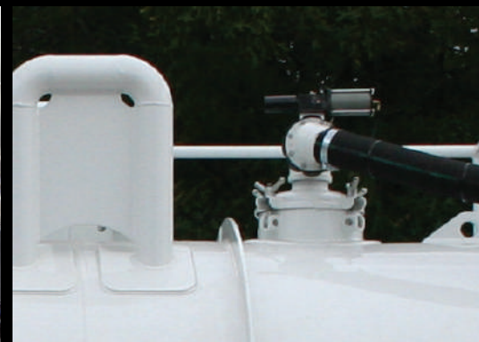
Emergency Shut Off
